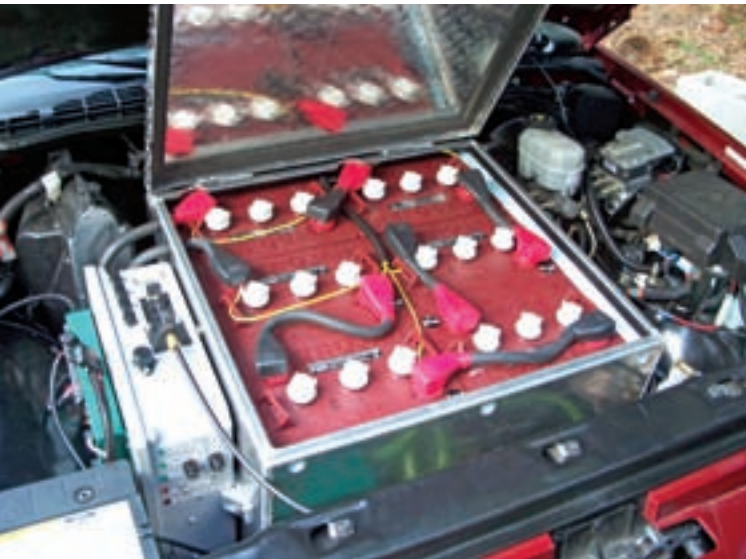
Above the drive motor— six T-145 lead-acid batteries and the control box, mounted to the left of the batteries.
